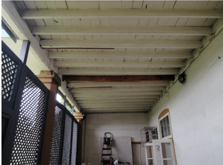
Figure 3. Show the suspended floorboards which have received repairs/restoration works in such a way that follows the existing construction method. This causes minimal disruptions to the character of the heritage building and was deliberately left unpainted to aid easy identification and appreciation of restorative efforts. Source: Author 2022.
