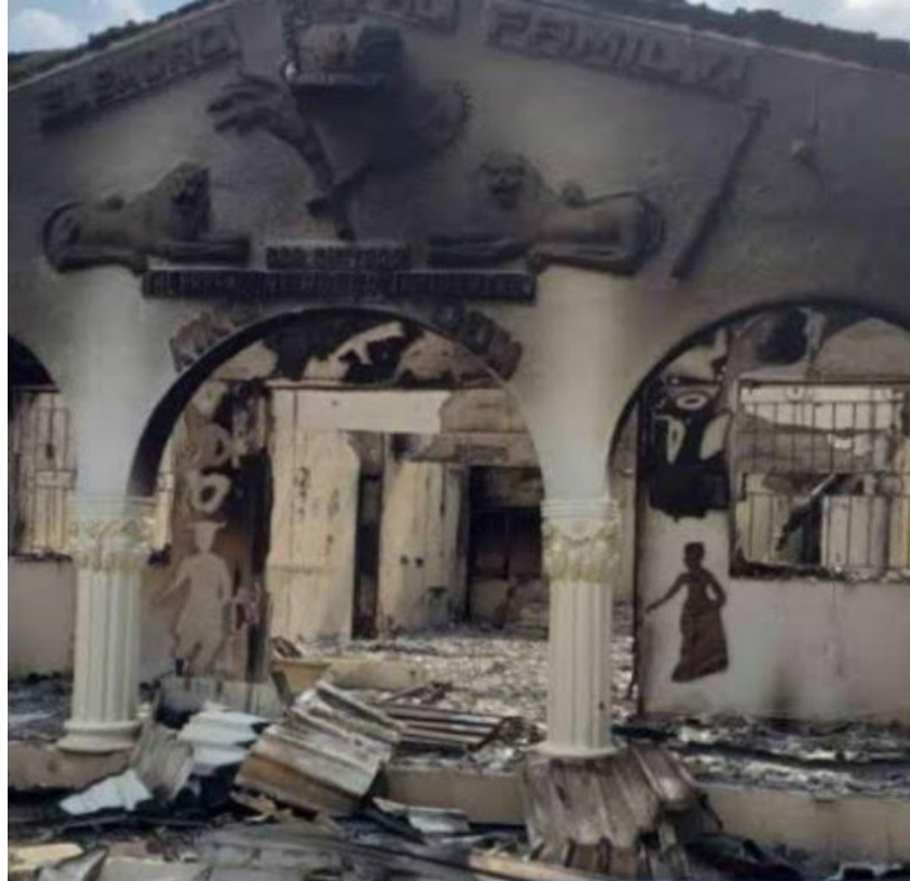
Figure 6. Pictures showing some of the damage to the building during the ENDSARS protests. Source: (Unini, 2020).
