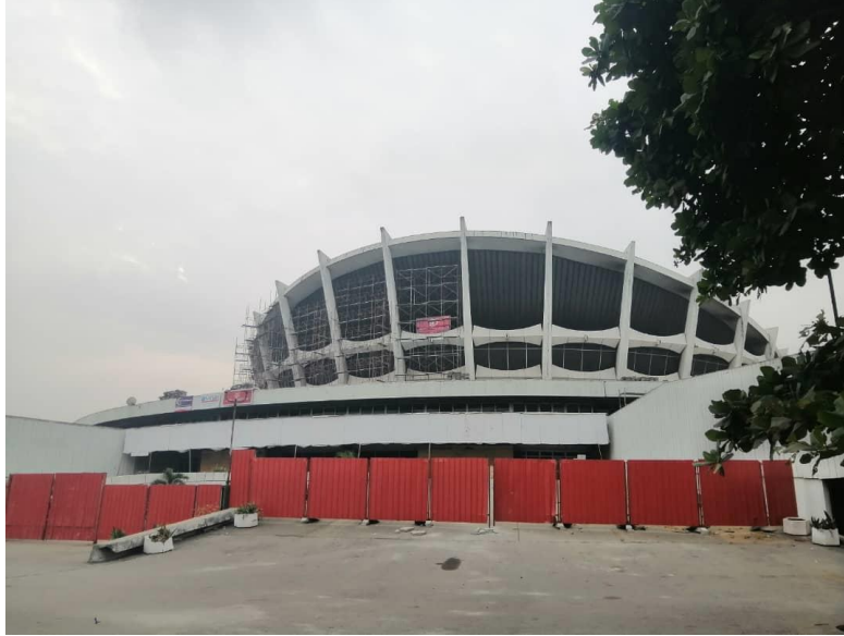
Figure 5. Exterior view of the Building cordoned off for the on-going renovation. General Comments: During the authors visit, the Building had been concessioned in 2020 by the Central Bank of Nigeria and the Bankers Committee and was under renovations. No access was granted to the premises for new internal pictures to be taken. Source: Author 2022.
